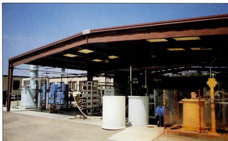
Advanced Wastewater Treatment - Filtration, Reverse Osmosis, and Activated Carbon Pilot Facility
