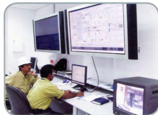
المرحلة السادسة Control Center at Administration Building
